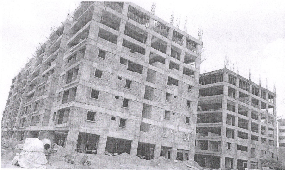
Block C2: Sixth Floor level slab concrete casting completed. Shuttering and Barbending work for 1 st half of Seventh Floor level slab 80% completed.
